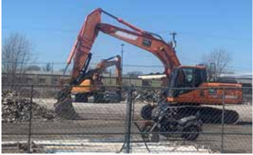
Excavators clear debris at the site of Afena Federal Credit Union's new corporate headquarters.
